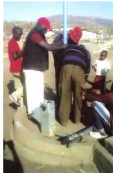
A new pump installed in Steiloop.
