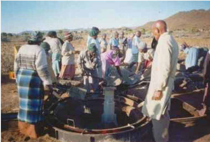
Men and women are learning how to construct a borehole in the Limpopo province.
