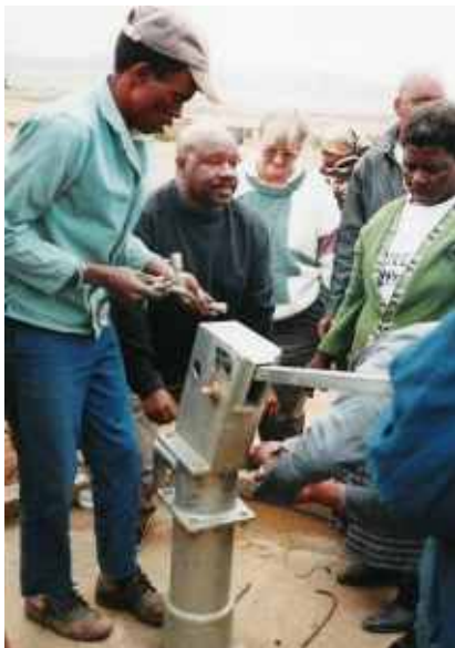
Borehole pumps are being maintained.
